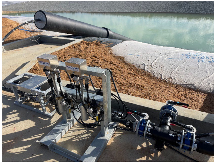
Image 1: Airwell leachate pumping system
