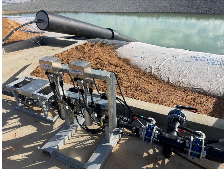
Image 1: Airwell leachate pumping system
